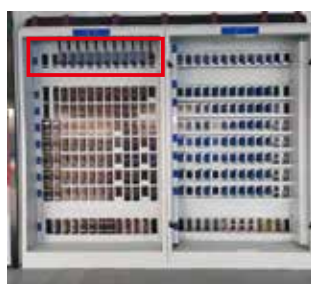
(b) 工厂化组合柜配线及架间配线 (b) Factory fabricated wiring of combination cabinet and between racks
